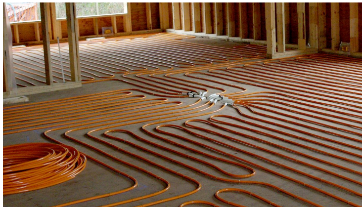
Figure 8: Image of an installed hydronic radiant heating system[6].
